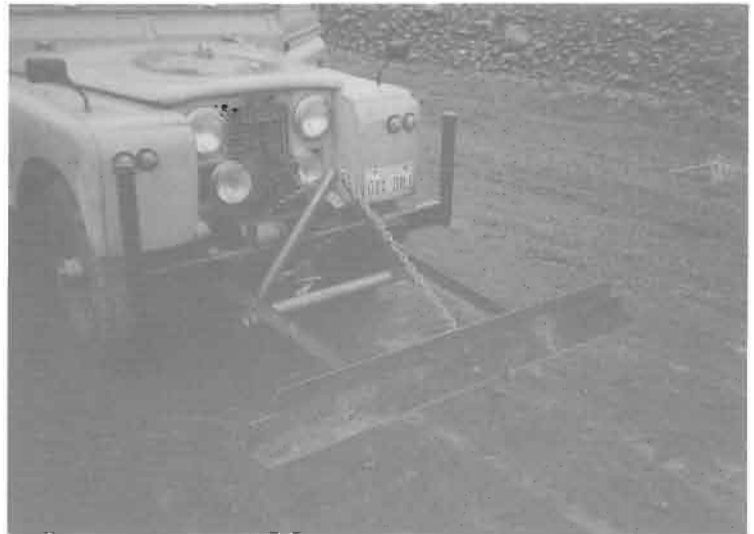
J. Ousterhout put together this push Blade used for re-filling their powerline trench. The winch runs it up & down.
