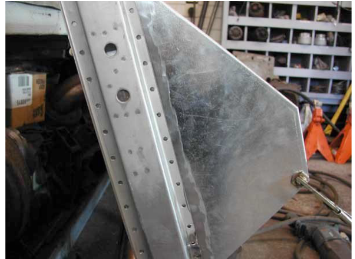
(Figure 11) With the door post accurately replaced the footwell can then be assembled. Here you can see the replacement door post has been drilled and the galvanizing ground away in preparation for welding the two panels together.
