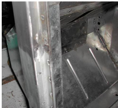
(Figure 10) With the old post cut off the jig is used to position the
