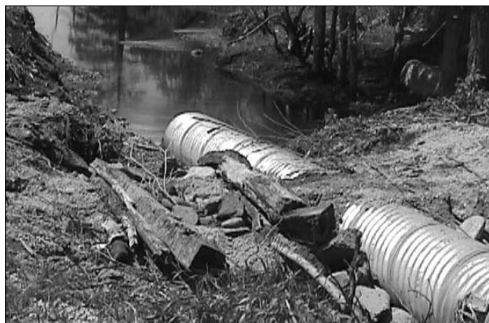
The newly reconstructed entrance to the railway bed from the Deacon's Photo: Kevin Willey
